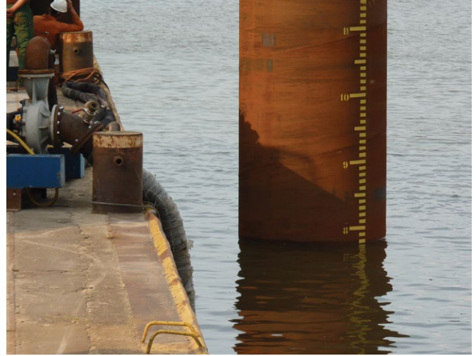
The series of tests were successful and provided more insight into the pile driving properties and underwater noise emissions of the technology
